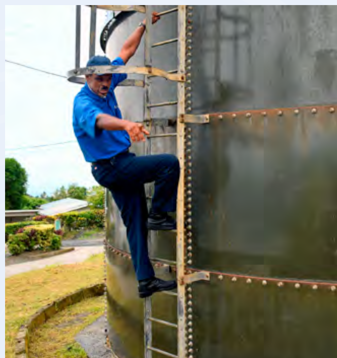
A WASCO employee inspecting a water storage tank at La Haut village.
